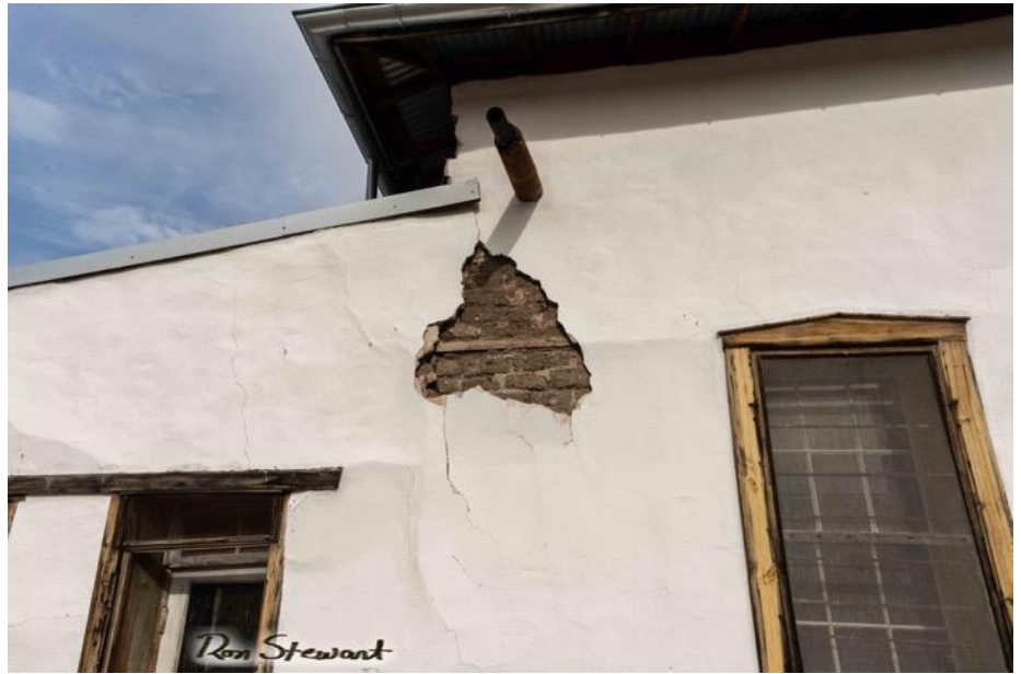
Here, you can see the cracking and crumbling plaster on the front of the Mercantile. Anyone want to donate some money to get it fixed?
