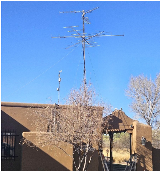
Antennas installed on a mast at the Casa de San Pedro by SABO. Copyright 2025 Southeastern Arizona Bird Observatory.
